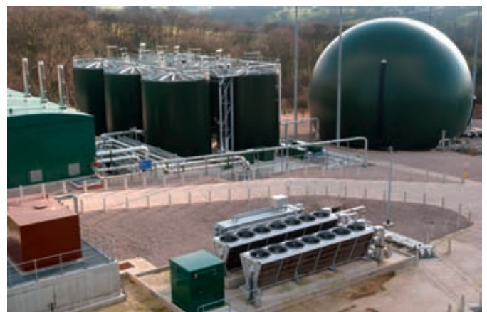
Blackburn waste water treatment works
